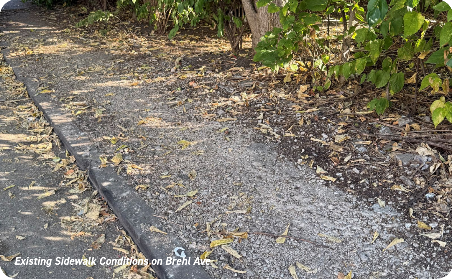
Existing Sidewalk Conditions on Brehl Ave
